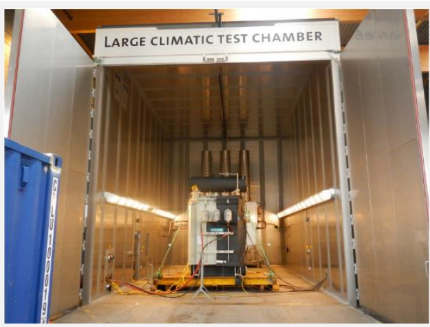
Large Climate Chamber +/- 60°C 10.6 x 7 x 8m >150 ton equipment 5% to 95%RH Ice-spray testing www.owi-lab.be
