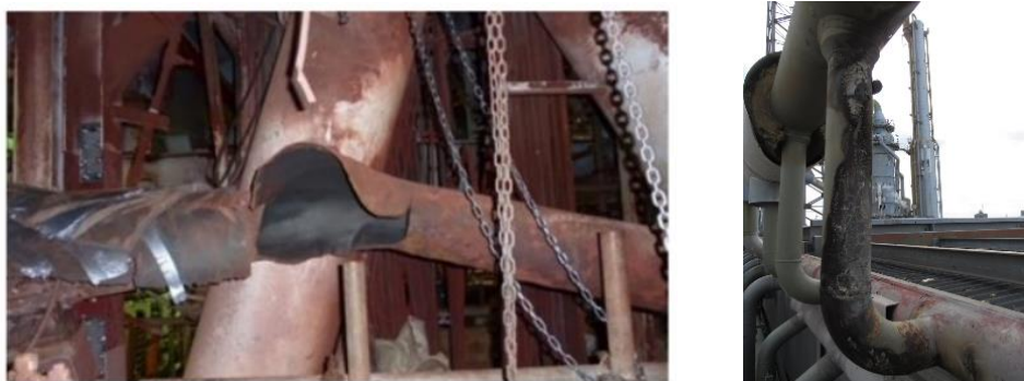
Figure 3. Examples of preventable serious failures if reliable inspection schemes had been used.
