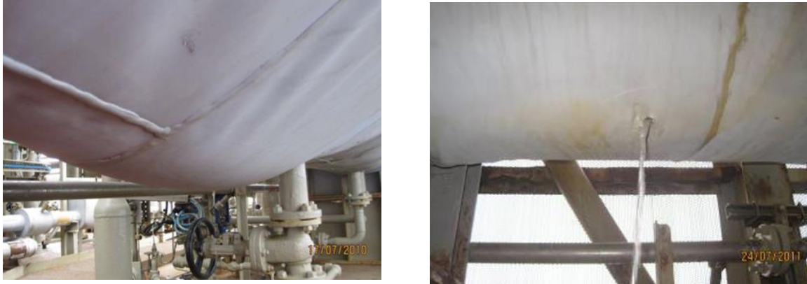
Figure 6. Tell-tale signs of bulging in a flexible non-metallic product due to water accumulation
