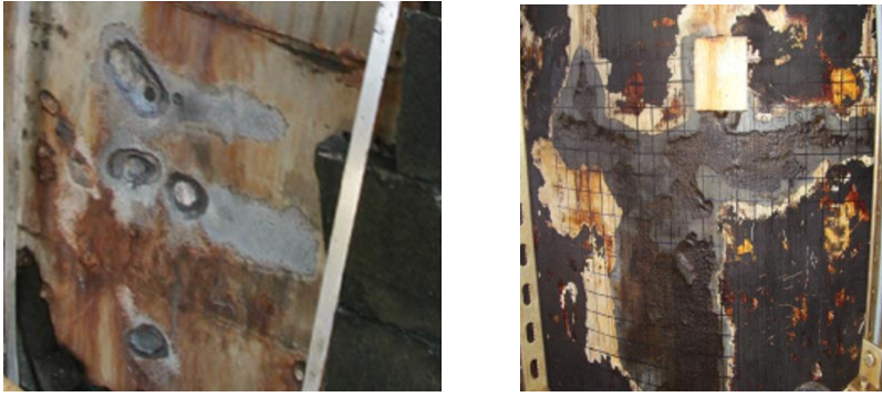
Figure 4. Examples of early severe CUI (>10mm loss in 6-10 yrs) in unusual locations associated with use of adhesive with closed cell insulation for equipment operating at elevated temperature.
