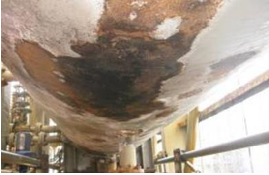
Figure 5. Example of TSA coating degradation under insulation after 17 years at 100°C
