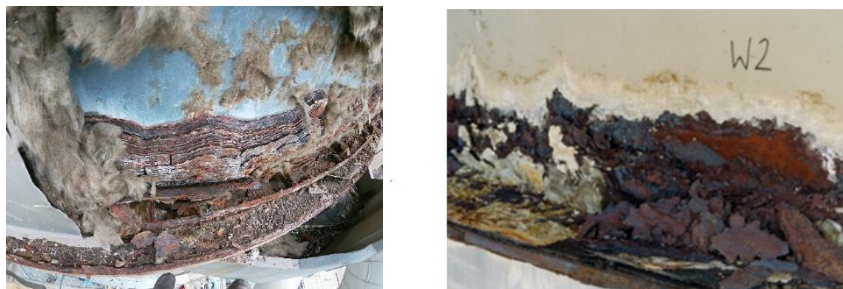
Figure 2, CUI of column support/stiffener rings to CUI Plant A (left) through-wall leak 2020 age 20 years. Plant B (right) severe CUI 1999 age 5 years.
